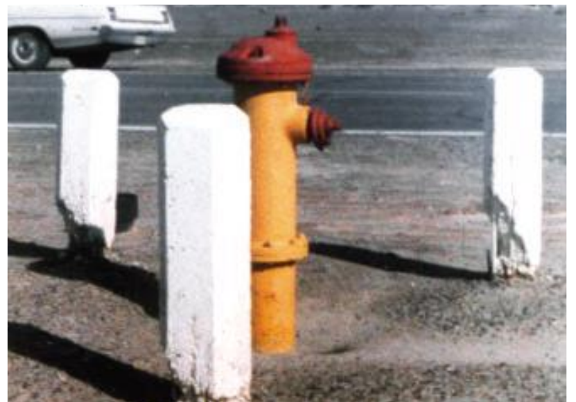
► Fig. 3: The bases of these concrete posts have suffered from sulfate attack (Portland Cement Association, 2002)
